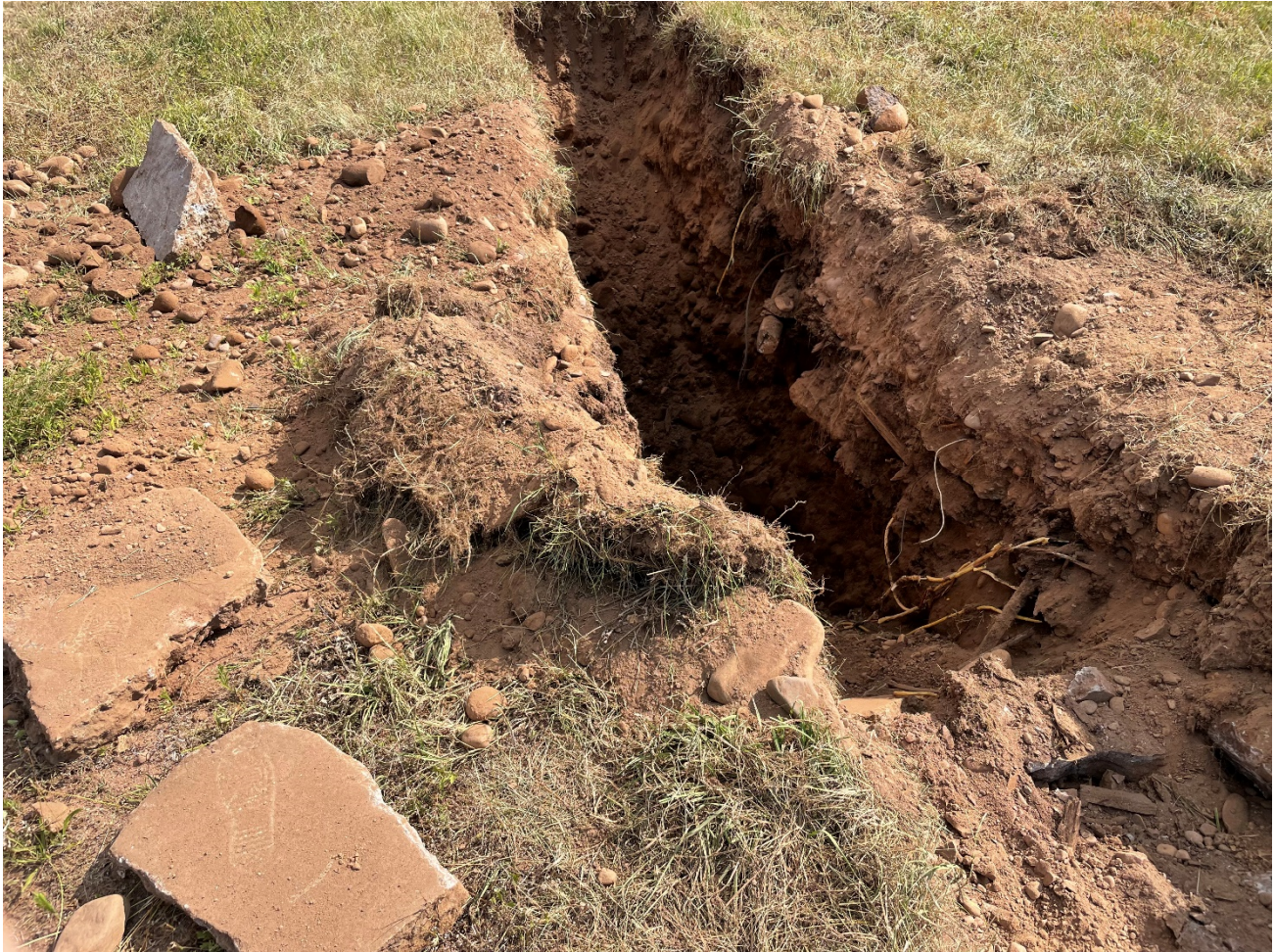
Photo 4: TP-27, located in the southern portion of the investigation area. Note inactive electrical lines and broken up concrete from the former barn.
